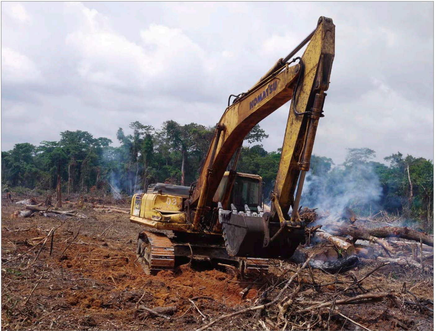
Figure 1. Rainforest in the Congo Basin being destroyed for a Chinese-funded road construction project (photo by William Laurance).
